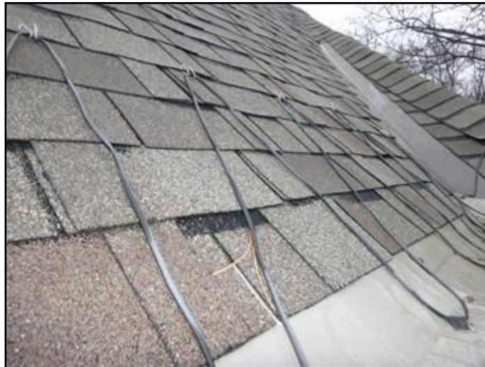
ice melter cables noted
