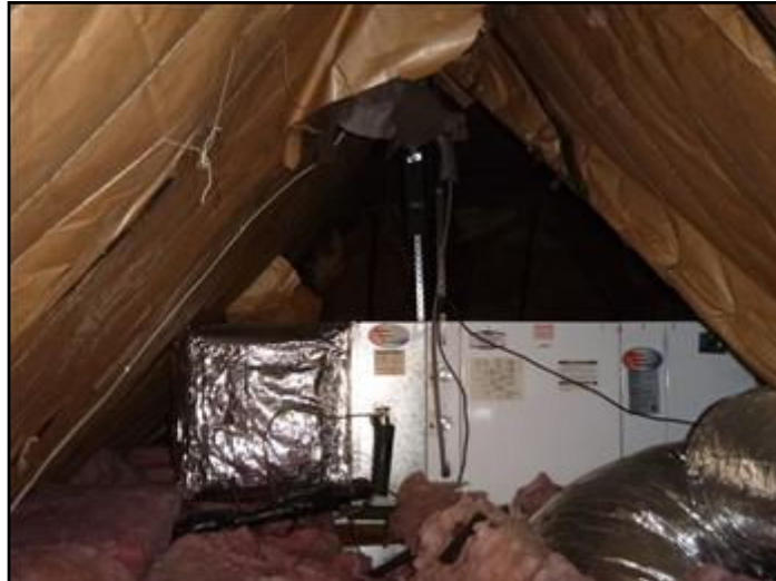
A/C air handler in attic space
