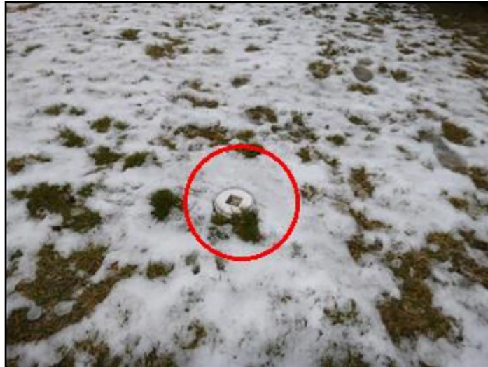
newer plastic clean-out noted at front yard
