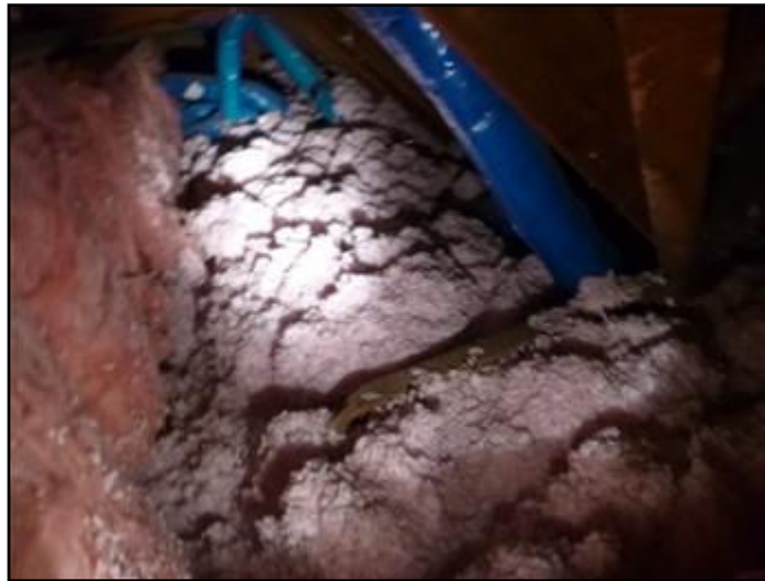
Some evidence of vermin activity was noted
