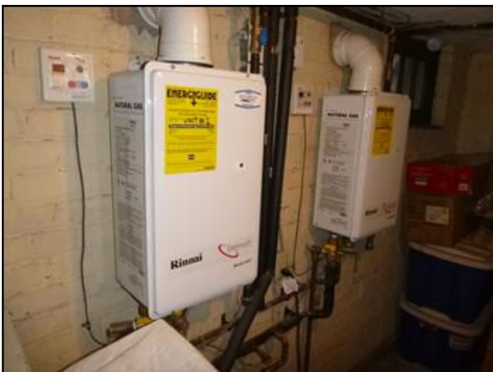
two tank less water heaters are used
