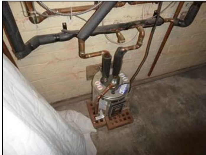
small storage tank
